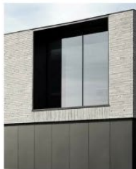
MT1 METAL FINISH TYPE 1-BLACK Steel metal mounted to large brick openings
