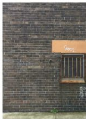
PF1 FACE BRICK TYPE 1 Existing brick facade to be retained For ease of existing brickwork Research to match for re-building the front apartment facade Research to match for proposed ground levels along with street level boundaries
